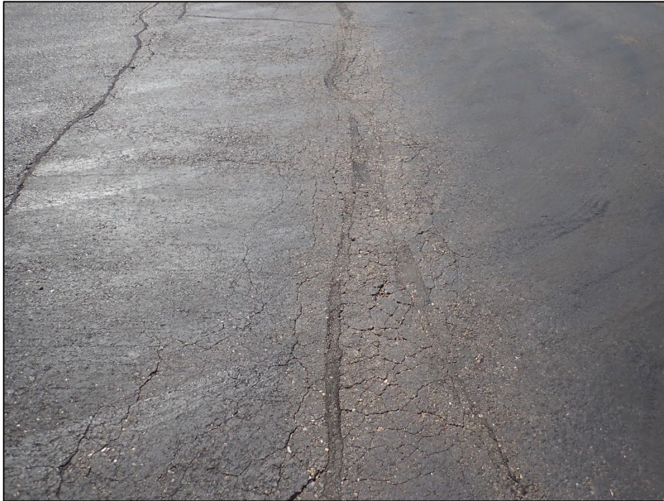
TW-03-19: Alligator Cracking
