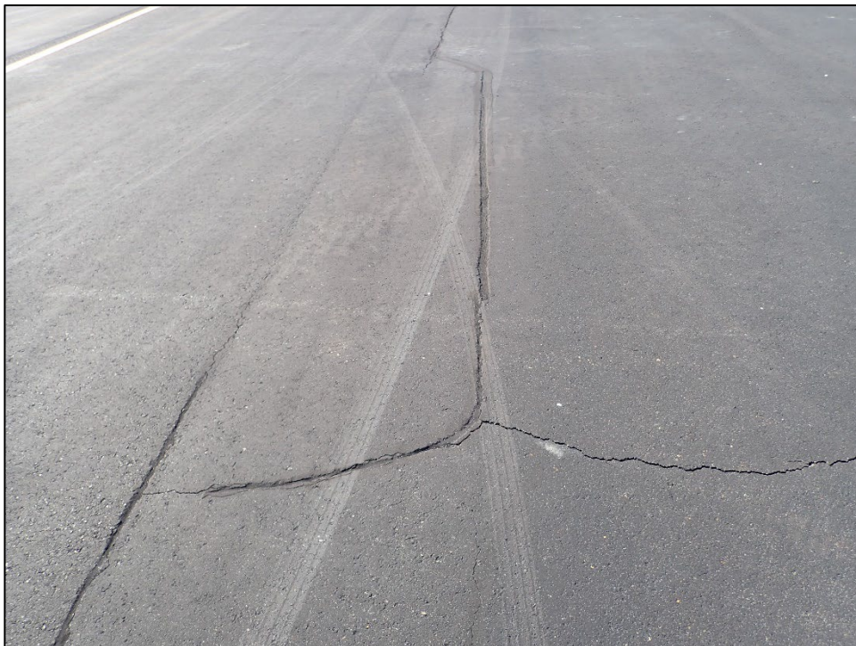
AP07-13: L&T Cracking
