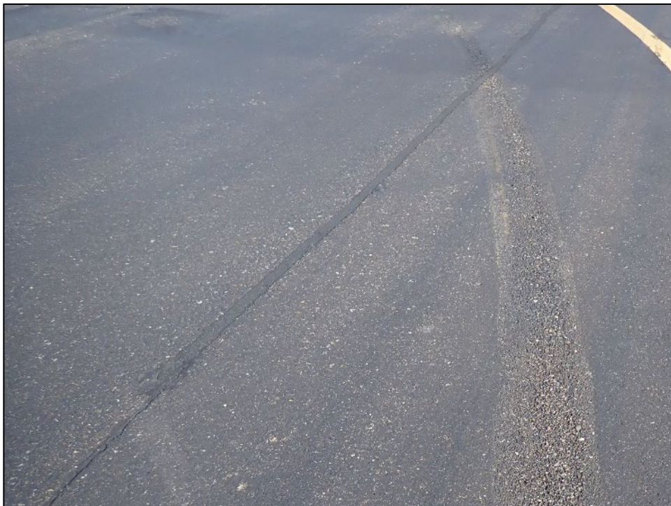
TW-01-07: L&T Cracking
