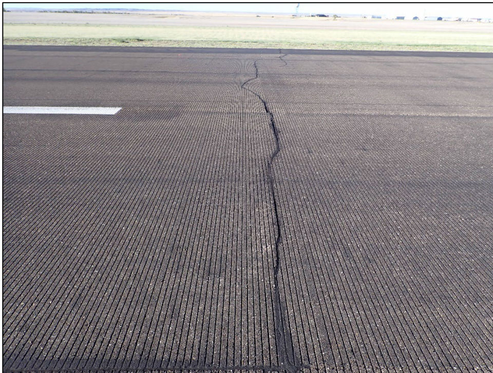
RW12-15-52: L&T Cracking
